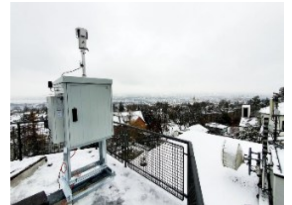
MeteoSwiss SwisensPoleno roof location in Zurich. Source: MeteoSwiss
